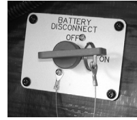
Battery Disconnect Switches
